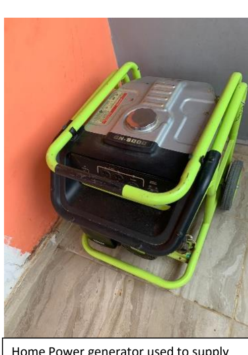
Home Power generator used to supply energy during power outages
